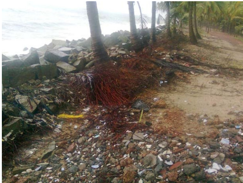
FIGURE 8: DAMAGED SEAWALL DUE TO COASTAL EROSION IN KANNUR DISTRICT
