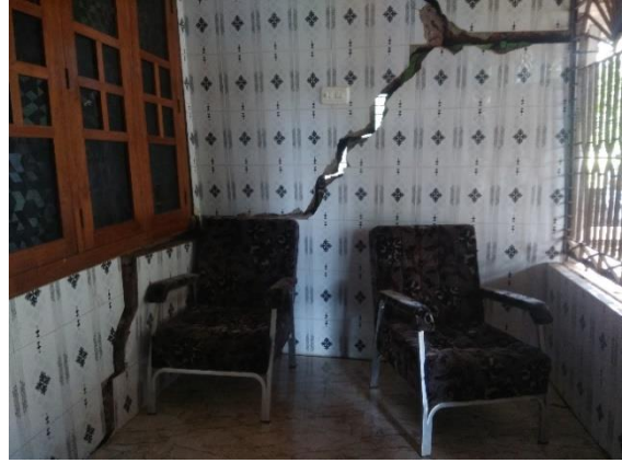
Figure 18 Cracked wall of Abdul Rahims house
