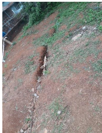
Fig 3 Fissure extending to eastern limit
