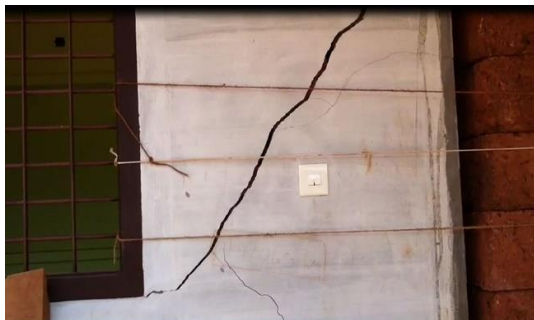
Figure 12: Zainudins house Cracks on the wall
