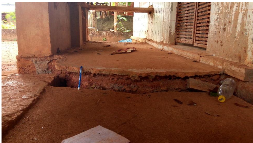
Figure 4 Ground fissures displacing the basement of the Abdul Rahim's house
