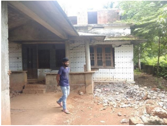
Figure 17 Damaged house of Abdul Rahim
