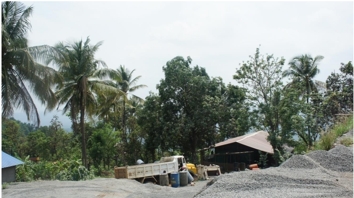
Photo 6: Stone crushing unit
