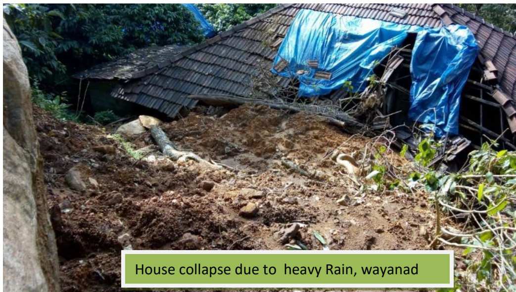
Soil washed out into house at Peruvanthanam village
