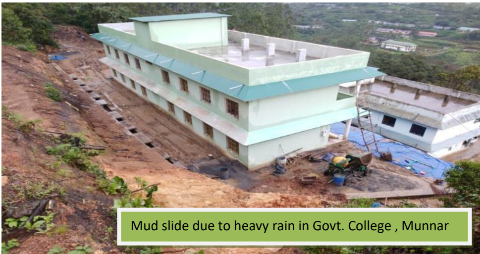
Mud slide due to heavy rain in Govt. College , Munnar
