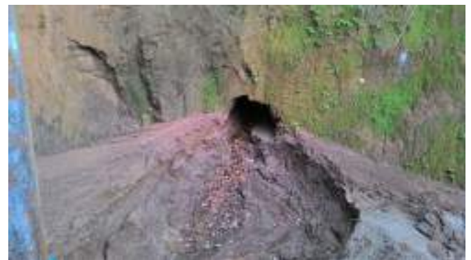
Fig.3. Soil piping in Muttill Mala, Wayanad
