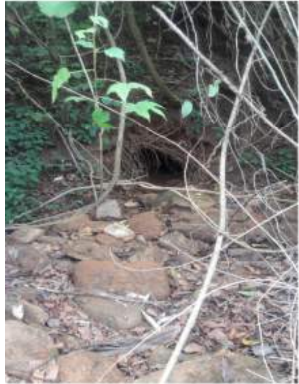
Fig.9 Piping formed at Puthenkadu
