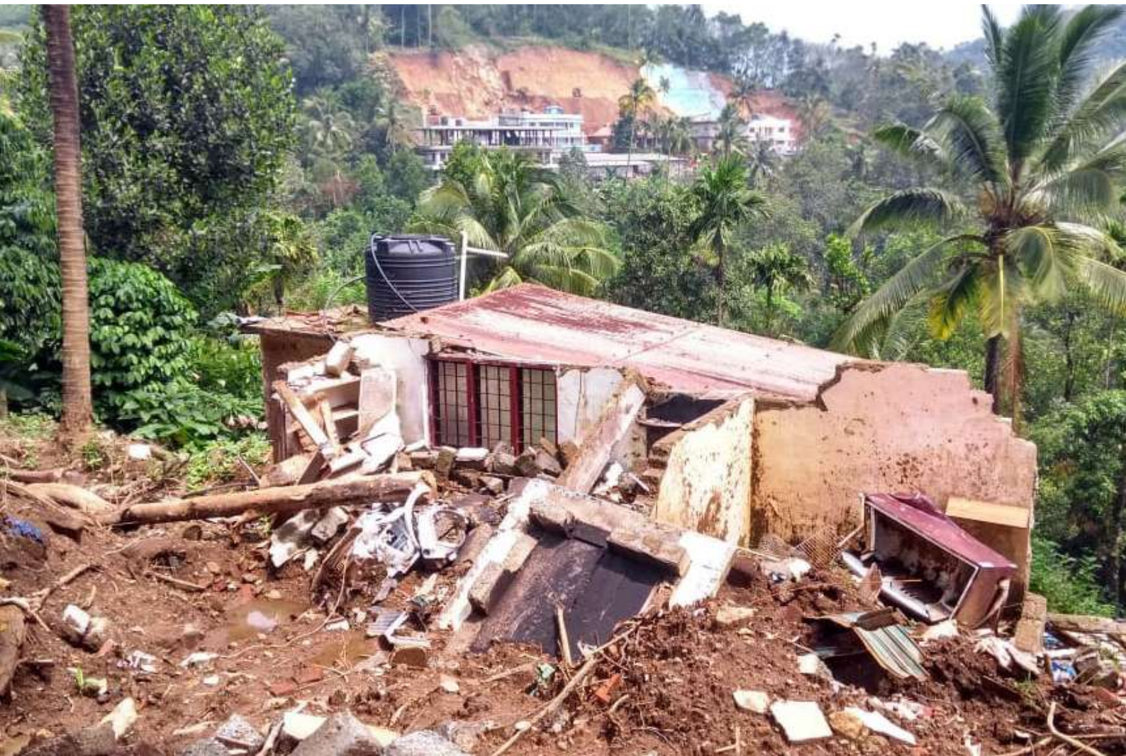
A collapsed house in landslip killing three members of a Dalit family, Cheruthoni, Idukki | CSSC
