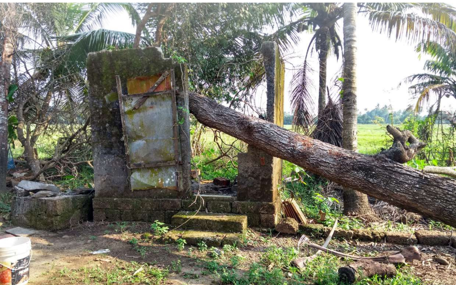
A toilet, collapsed at Ezhumamthuruthu | CSSC
