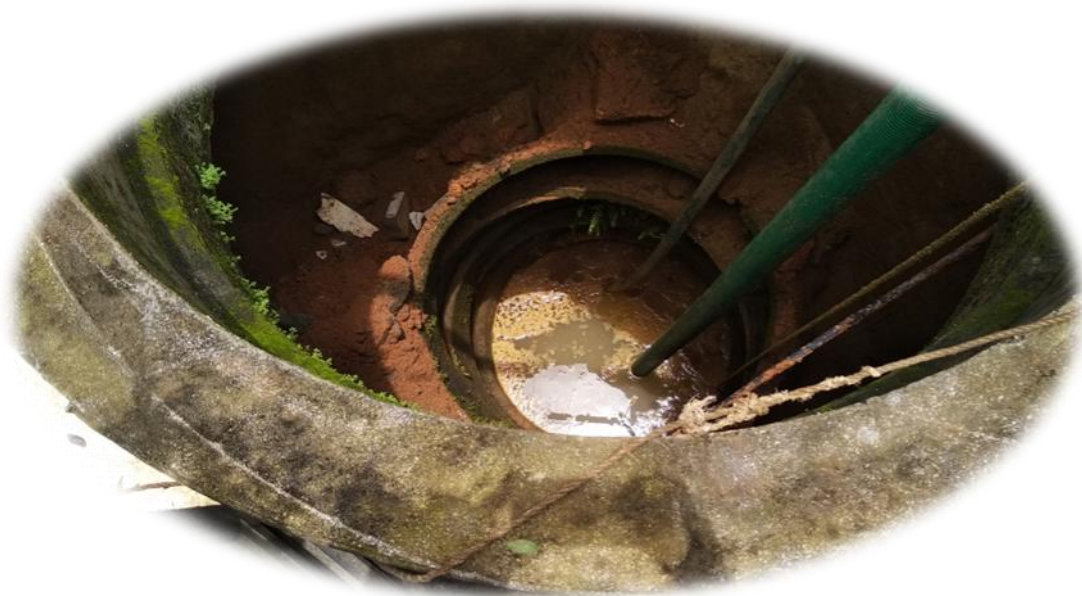
Destroyed Well due to Flood
