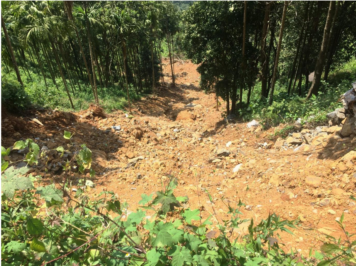
Plate 12: The scar of the failure starting towards valley from the road edge.
