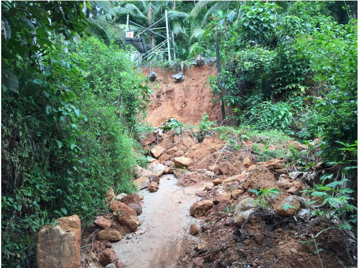
Plate 14: Slump due to soil piping in Chembattamel
