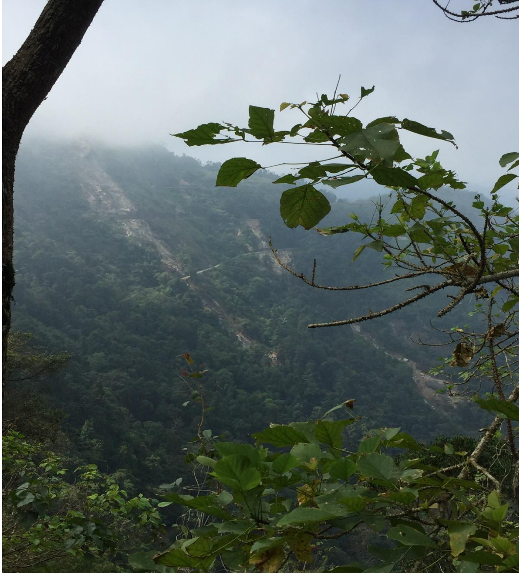
Plate 11: A view of series of slope failures in near Kakkayam Dam site.
