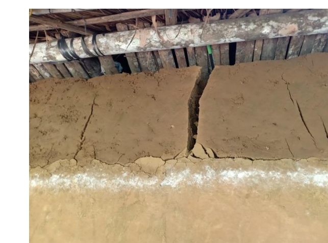
Cracks at the top of wall
