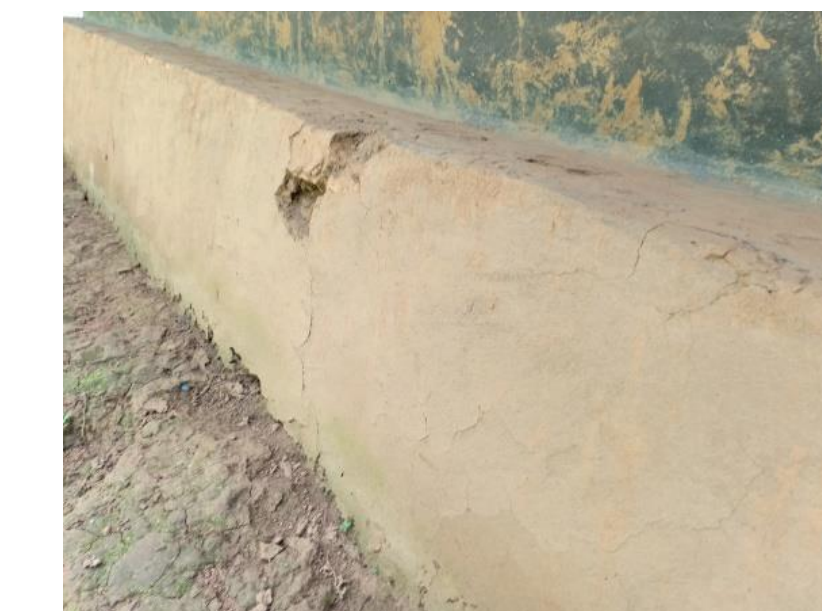
Damages on the foundation
