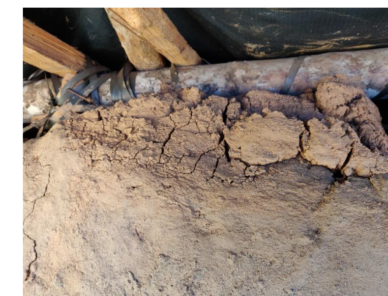
Cracks on mud walls
