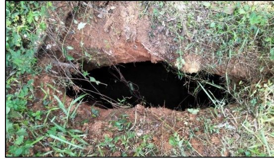
Figure. 4.11: Vertical cut slope made for house construction along the roadside where the roof of the tunnel collapsed
