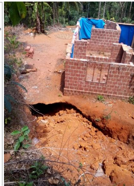
Figure 5.2: Damaged foundation in the study Area (Sankar 2015)
