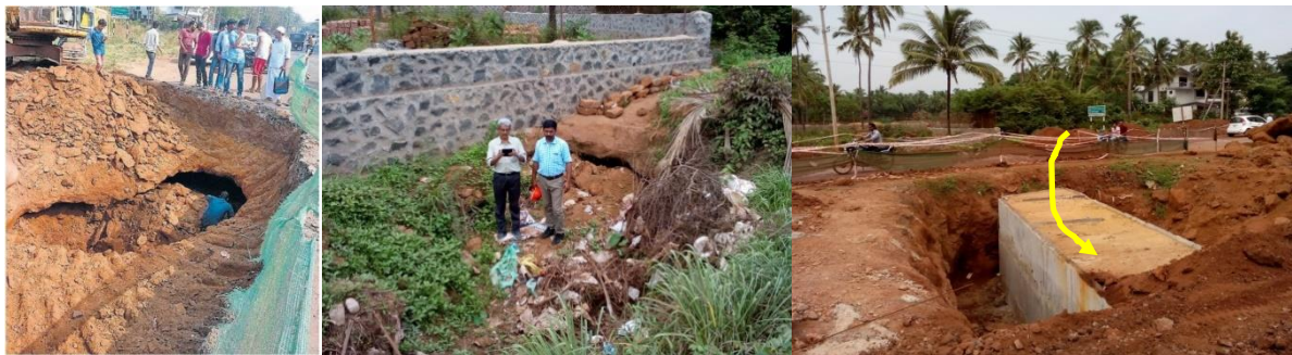
Figure 4.28: Soil piping incidence occurred in State Highway Pallikkara, Kasaragod District
