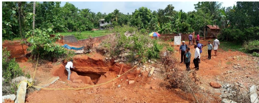
Fig 1.1 Land subsidence occurred due to soil piping in Kottaykkal, klari in 2018
