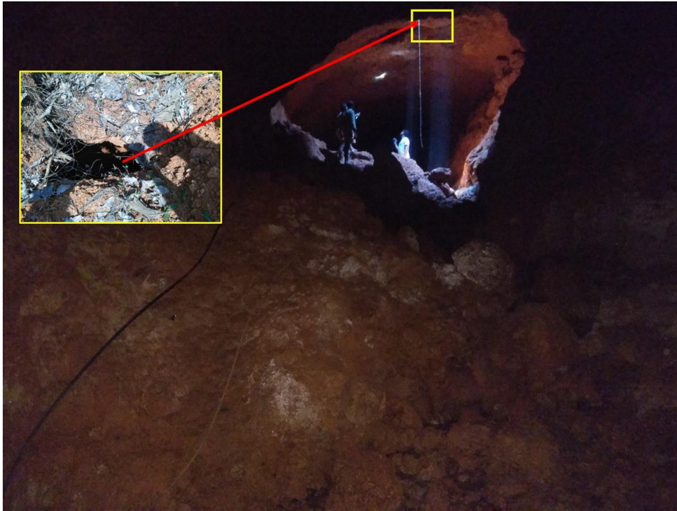
Figure 4.18: Cavity formed below road at Kizhakanodi
