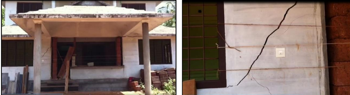
Figure 4.47: Showing the damaged house of Zainudin Paruthikunnen
