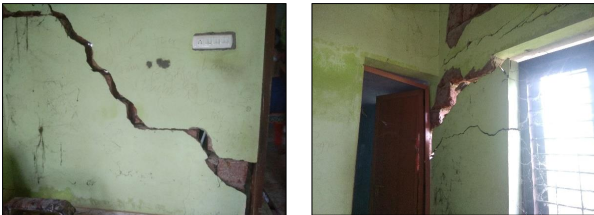
Figure 4.51: Cracks on the wall of affected house
