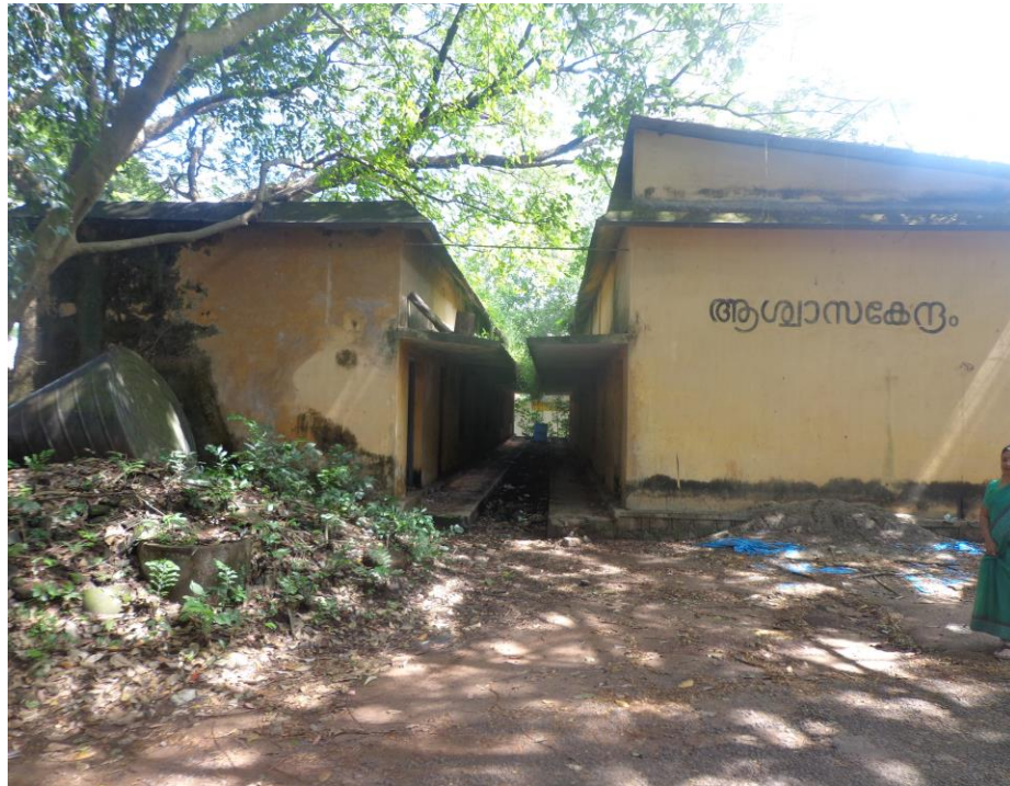
3. Dilapidated Shelters in the proposed site
