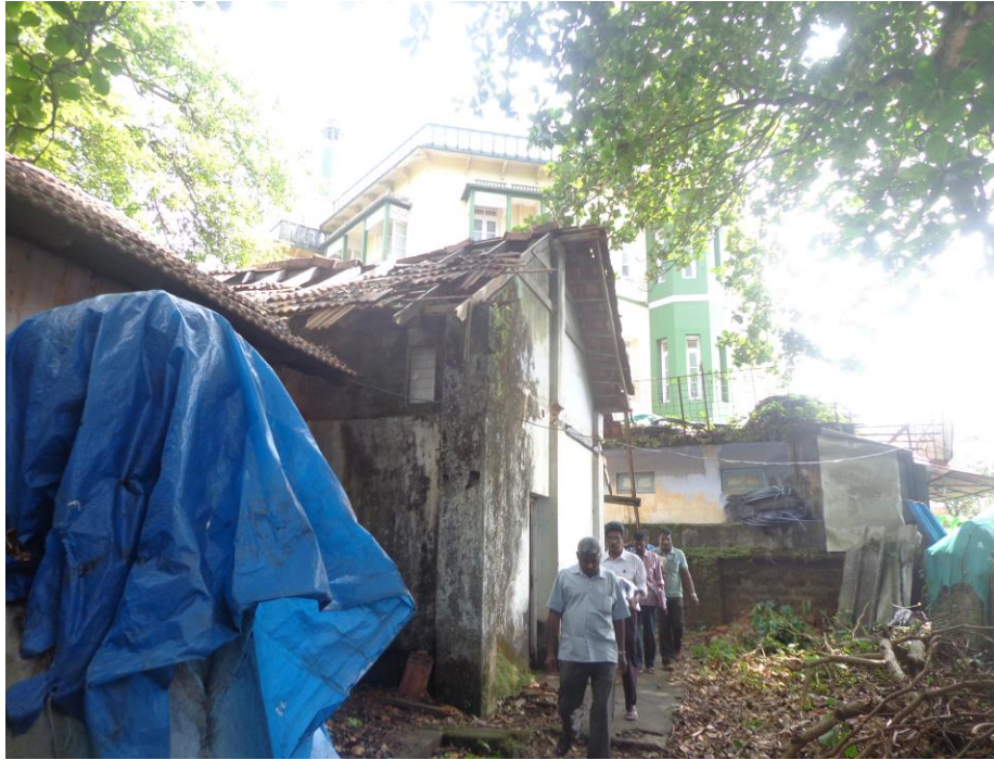
3:View of dilapidated building in the site. Mosque near to site can be seen.
