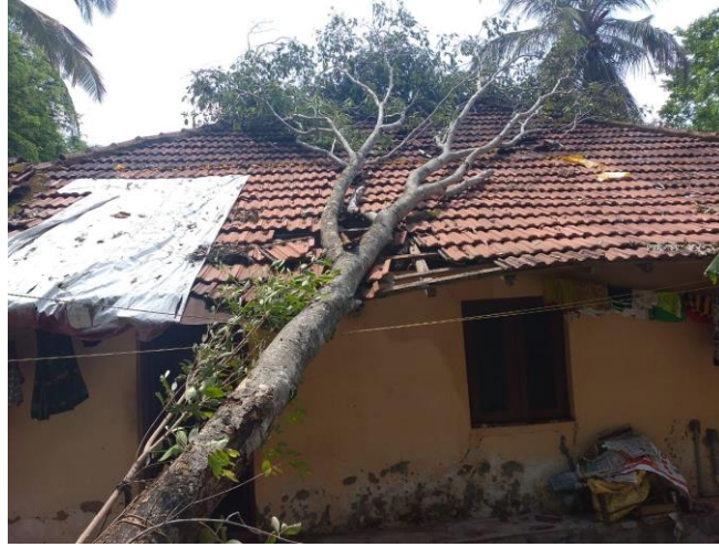
Figure 11. House damaged in Palakkad district ( Source: District Emergency Operations Centre, Palakkad)
