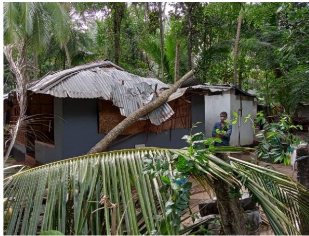
Figure 12. House damaged in Malappuram district ( Source: District Emergency Operations Centre, Malappuram)
